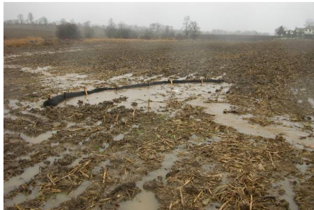
Figure 2. Filter sock accumulating water across a zone of concentrated flow during a rain in December, 2011
