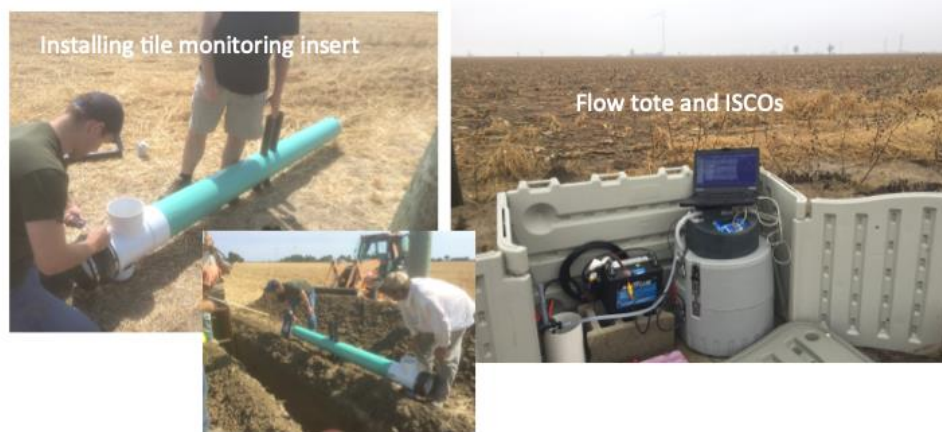
Figure 1.3. Edge-of-field water quality in the tiles was measured using area flow velocity sensors, and tile water quality samples were collected using auto-samplers (ISCOs).
